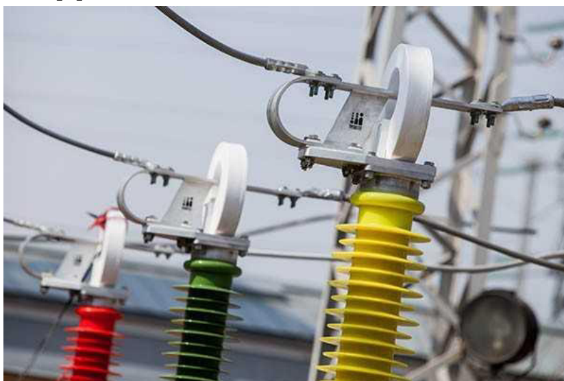
Figure 1 – Optical current transformers
